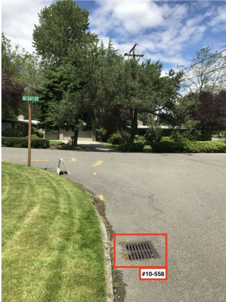
Facing N on the west side of 77th Ave SE, catch basin #10-558 in foreground.
