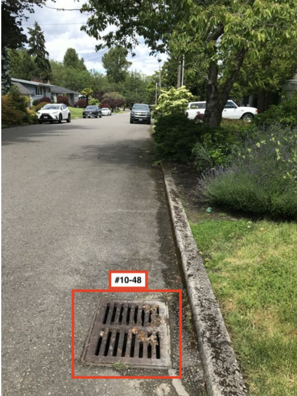
Facing N on the east side of 77th Ave SE, catch basin #10-48 in foreground.
